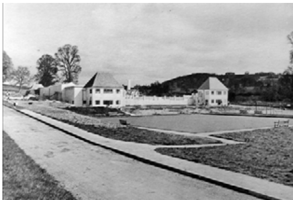
Above: The lido under construction circa 1937(Conservation Management Plan for Stratford Park and Museum in the Park. Oct 2006, pp.24)
