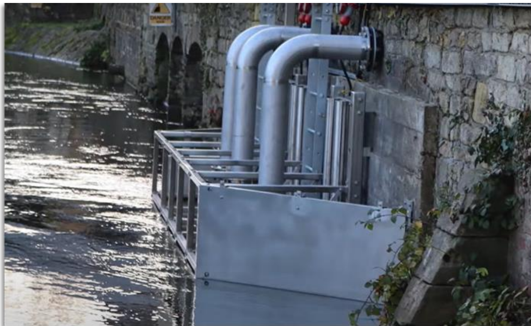
Water Source Heat Pump, Ebley Mill
