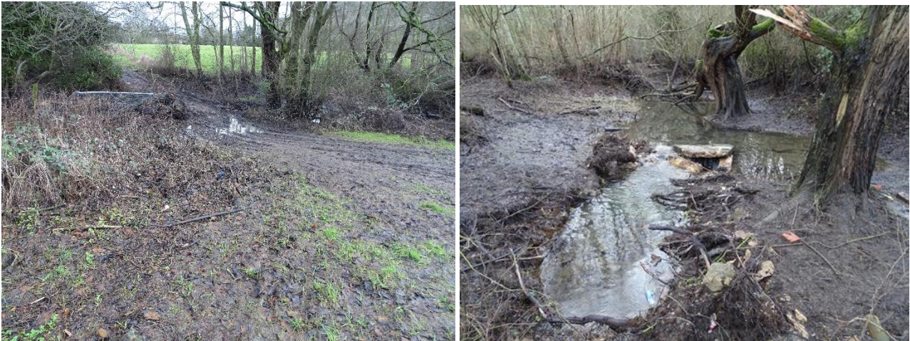
Further photos following drainage, showing the view of previously flooded area and stream and culvert entrance.
