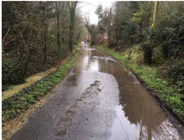
Flooding in Ryalls Lane - the ditches are full
